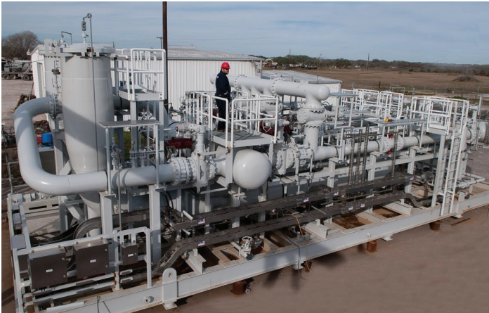
Metering and proving systems
